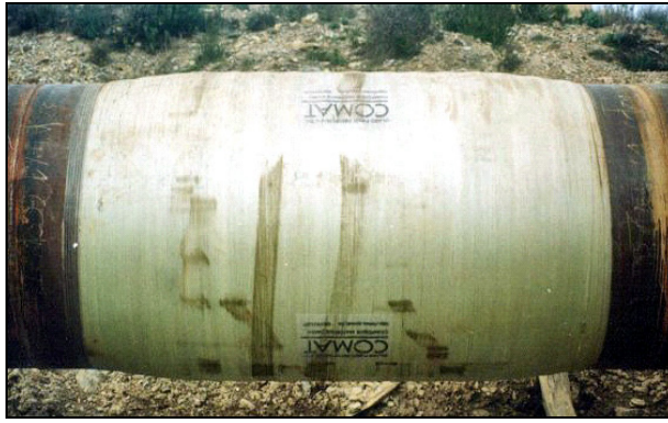
Figure 11. Composite CA section used in 2 nd full-scale DEMOPIPE project (CA provided by Europipe).
